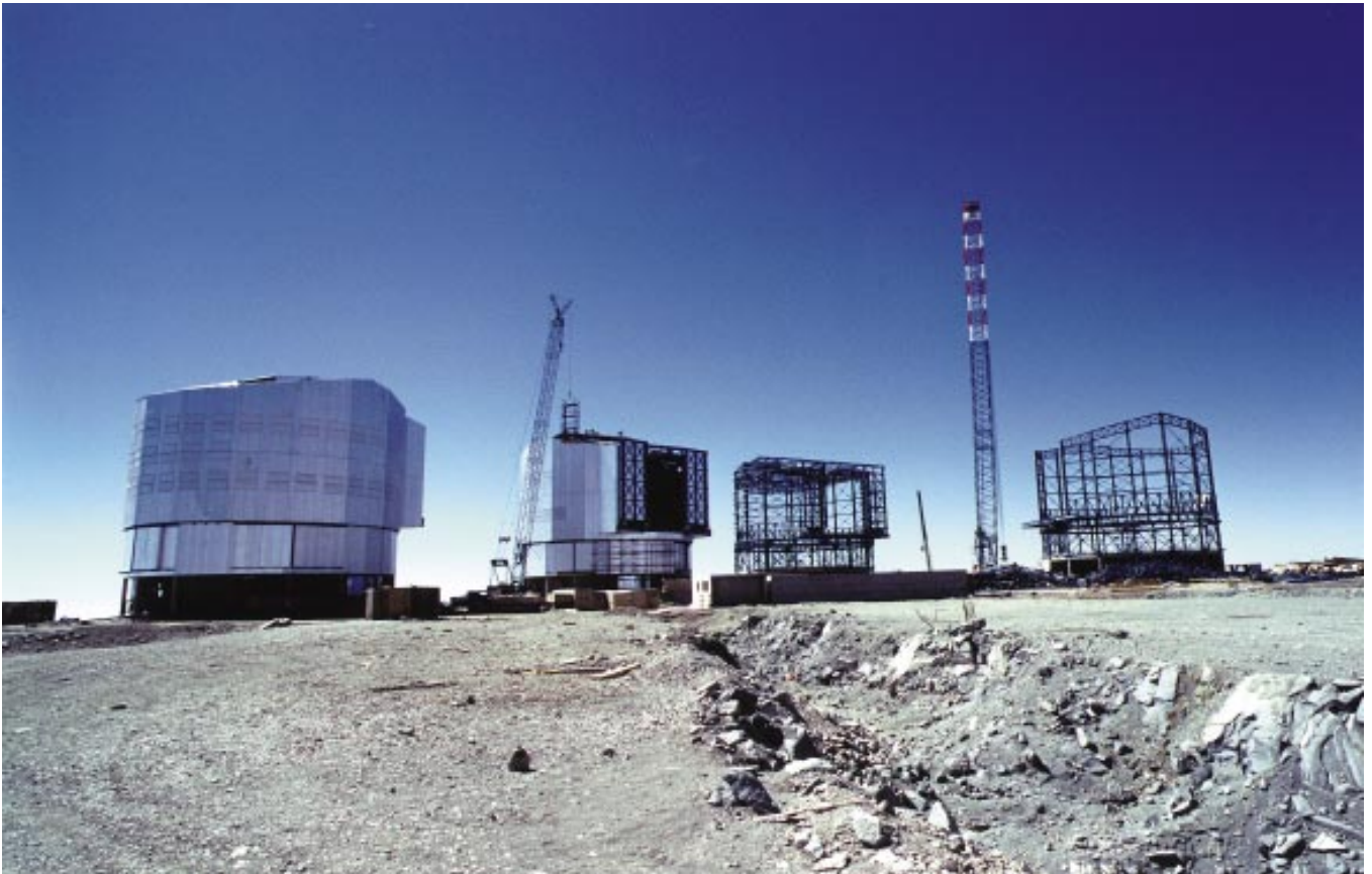
Figure 1 was obtained mid-October 1996 and shows the four enclosures at different stages of integration. No. 1 is complete, no. 2 is in the final stages of the implementation of the aluminium cladding, no. 3 is ready for enclosure cladding and no. 4 is in the final stages of steel erection which was completed the following day with the positioning of the roof using the 350-ton crane situated next to the dome.
