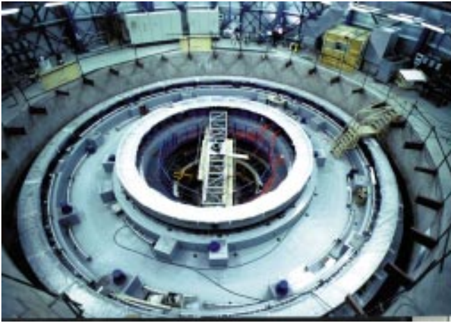
Figure 3 was taken inside enclosure no. 1 and shows the 2 azimuth tracks of the first telescope structure already in place and going for the final adjustment. The inner part shows the cable wrap in place and the beginning of the installation of the necessary connections. At the bottom of the hole the coudé rotating platform has already been installed.
