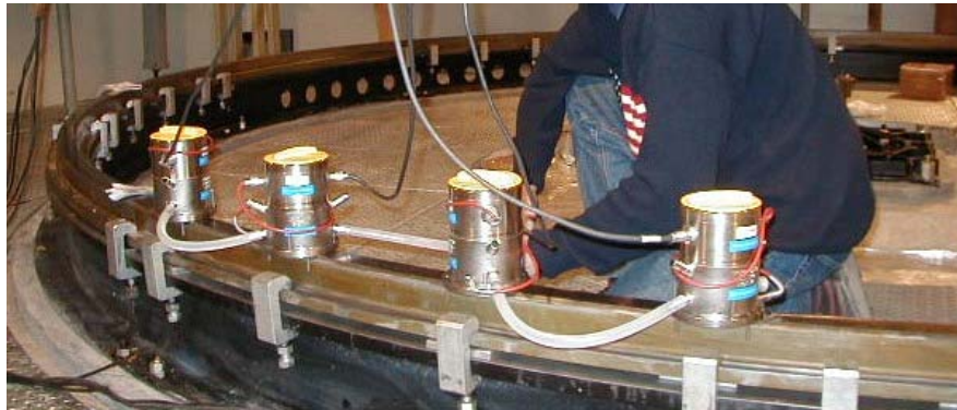
Figure 13-3: Azimuth tracks alignment metrology.
